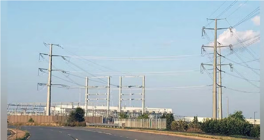
A large power substation in Data Center Alley, Ashburn, VA
